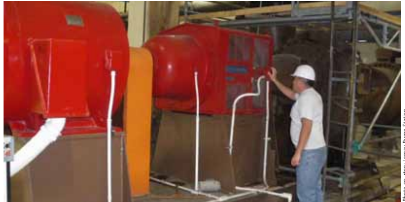
Photo courtesy Lemay Pump Station
